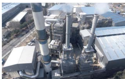
Changwon Enertec : Industrial Waste Treatment, Stoker, SRF Boiler, SRF Manufacturing, Steam Supply and 2.75MW Power Plant
