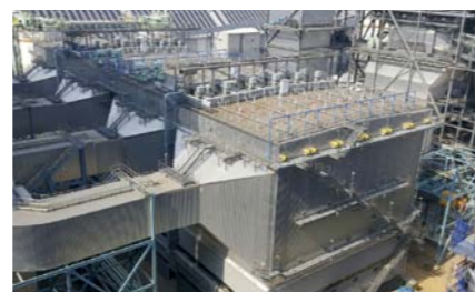
Shinboryeong Thermal Power Plant
