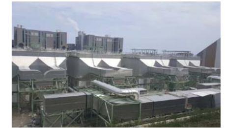
Samcheok Green Thermal Power Plant
