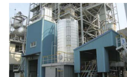
CFBC Boiler, LG Chem Company
