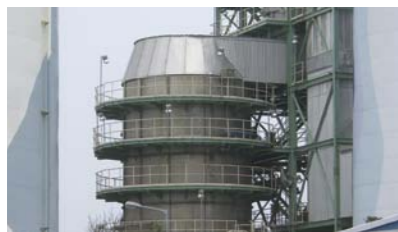
Jeju Internal Combustion Plant
