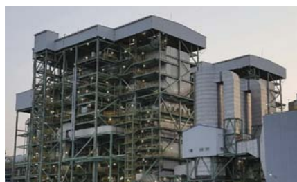
Saemangeum Power Plant
