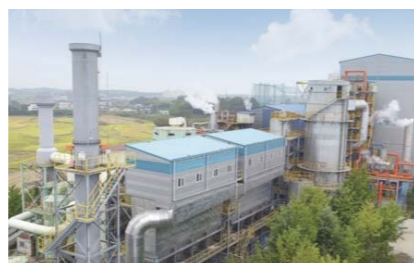
KC EnviroServices(Jeonju) : Industrial Waste Treatment, R/K+Stoker, SRF Boiler & Manufacturing, Steam Supply and Power Plant
