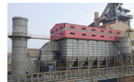
Krakatau POSCO Sinter Plant
