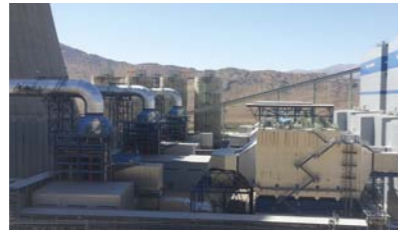
Tufanbeyli Thermal Power Plant
