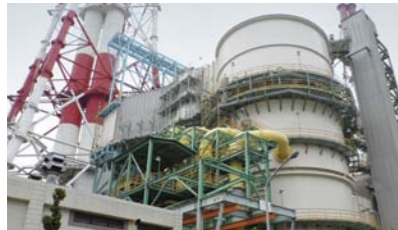
Hsinta Thermal Power Plant
