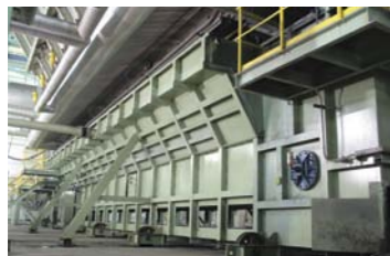
Bottom & Fly AHS, Dangjin Thermal Power Plant
