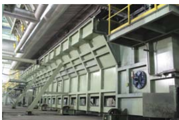
Bottom & Fly AHS, Dangjin Thermal Power Plant
