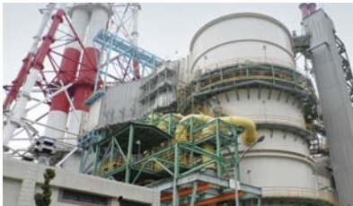
Hsinta Thermal Power Plant
