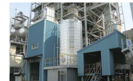
CFBC Boiler, LG Chem Company
