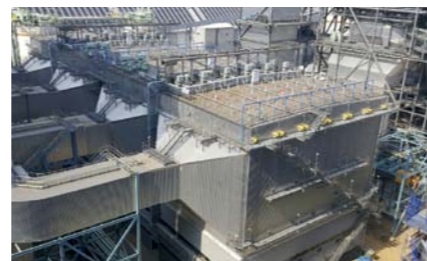
Shinboryeong Thermal Power Plant
